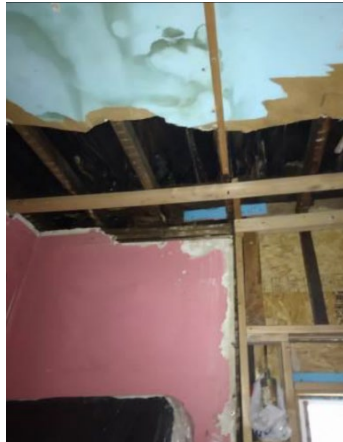
Ceiling damage from a leaking roof.
