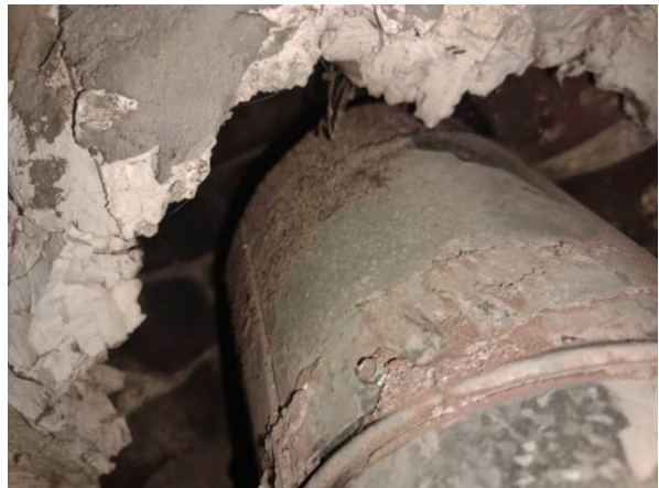
Figure 32: A flue terminating into a masonry chimney with no chimney liner.
