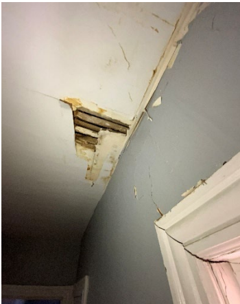
Ceiling damage from a leaking roof.
