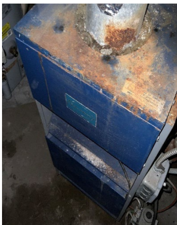
A deteriorated boiler at the end of its useful life.
