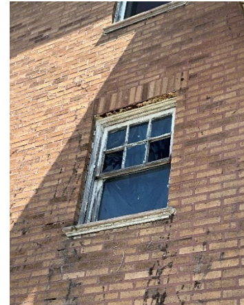
Broken window with deteriorated paint trim.
