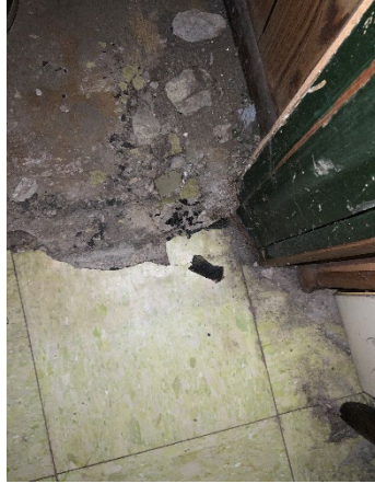
Cracked floor tile in a basement, likely containing asbestos.
