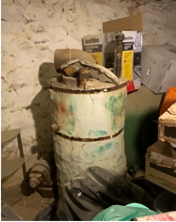
A disconnected water heater wrapped in asbestos.
