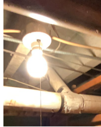
Asbestos pipe insulation on basement boiler pipes.
