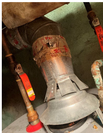
A dangerous, improvised solution to a disconnected water heater flue.
