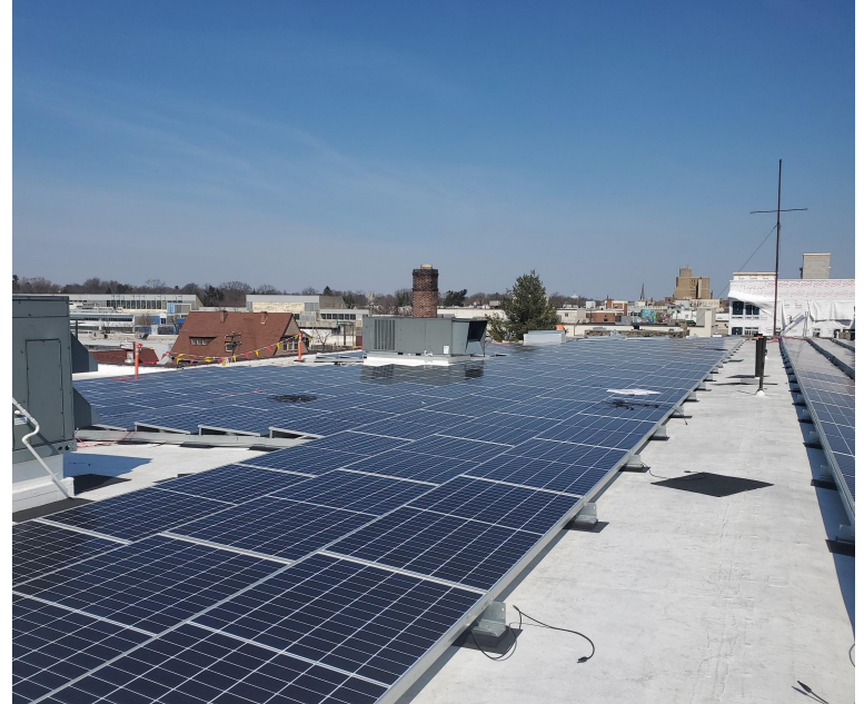
Solar on Olde City Day School, Germantown
